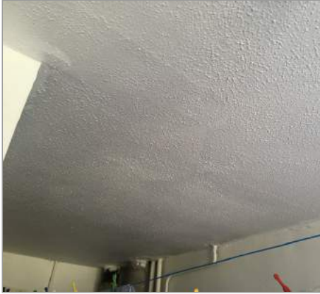
Photo - 26 Could contain asbestos
