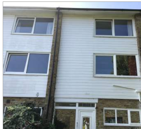
Photo - 4 Staining to front pier
