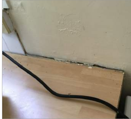
Photo - 53 Sealant required
