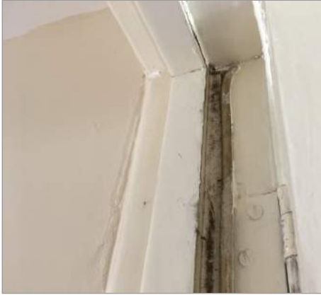
Photo - 66 Defective fire door strips
