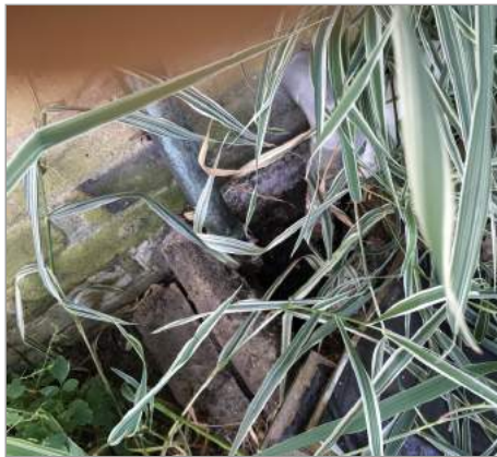
Photo - 83 Front gully
