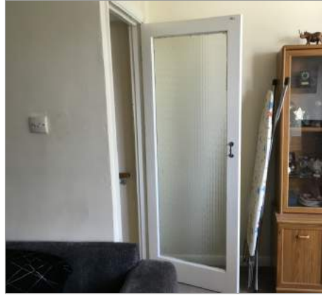
Photo - 59 Georgian wired door should be safety glazing
