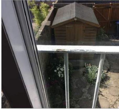
Photo - 14 Maintenance required
