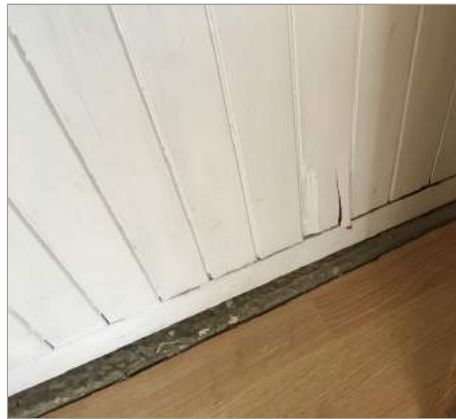
Photo - 65 Damage to under stair cupboard door
