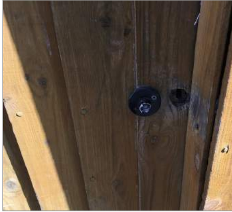
Photo - 93 Requires repair
