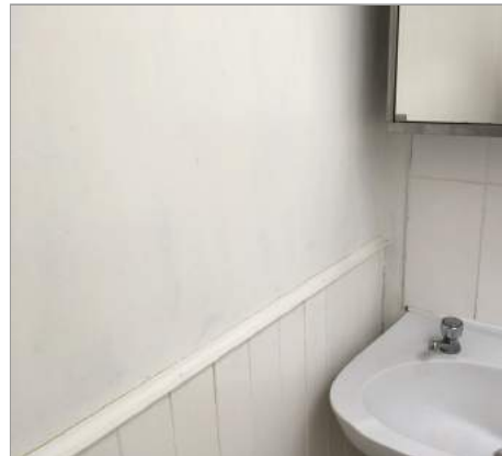
Photo - 33 Timber panelling is a fire risk
