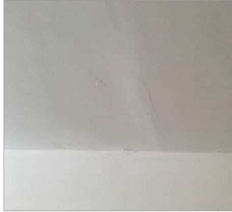
Photo - 27 Poor plaster skim patch up
