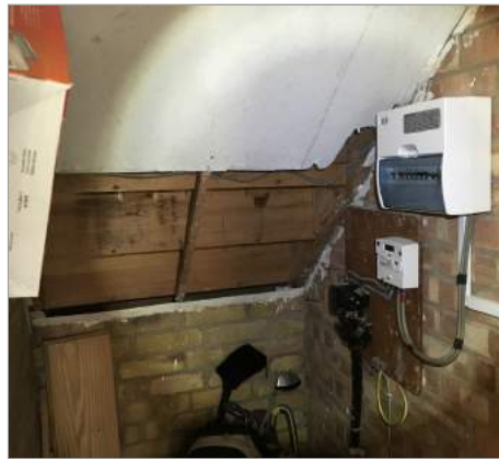
Photo - 61 No fire protection to stair under side
