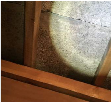
Photo - 24 Felt could be asbestos based?
