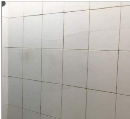
Photo - 32 Cracked tiles
