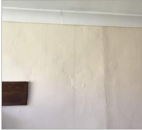
Photo - 38 Crack to ground floor wall
