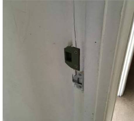
Photo - 55 Split to door frame lining
