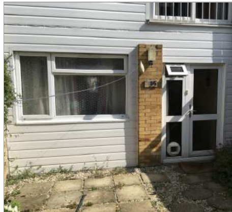
Photo - 12 Middle side pane to be confirmed as safety glazing. Back door key to be located and door tested to see if it opens
