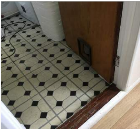
Photo - 60 Cat flap breaches door integrity. It should not be cited in a fire door
