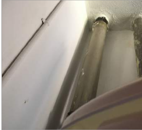
Photo - 81 Services should be boxed in in fire rated construction or fitted with fire collar to soil and vent pipe
