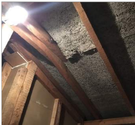
Photo - 20 Repair felt and find out what the material is before doing so.
