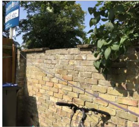
Photo - 92 Requires maintenance
