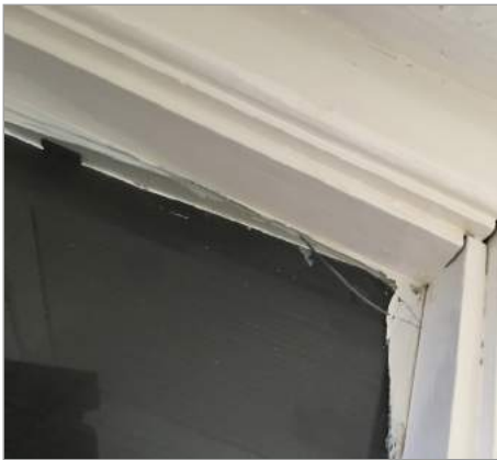
Photo - 64 Crack to door glazing to bedroom. It should be fire rated if on a protected stair
