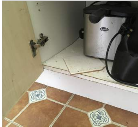
Photo - 51 Damage to cupboard
