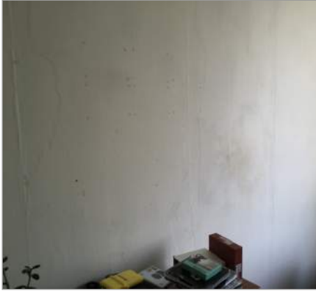
Photo - 34 Walls require making good, cleaning and redecoration throughout.
