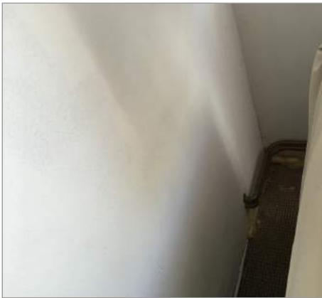
Photo - 47 Foam at bottom of wall
