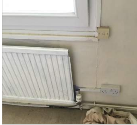
Photo - 39 Expansion contraction cracking
