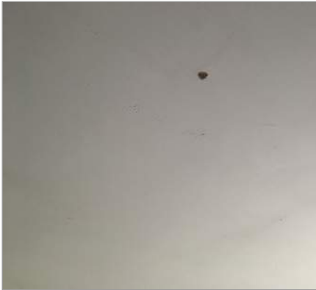
Photo - 28 Mechanical damage
