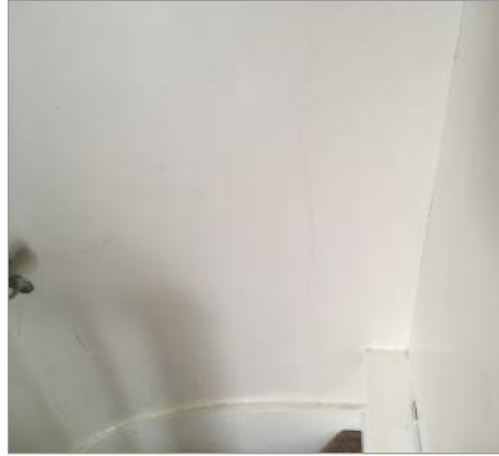
Photo - 35 Crack on second floor stair
