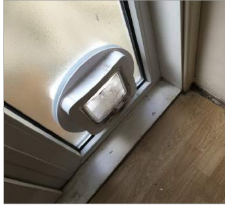
Photo - 46 Poor detailing
