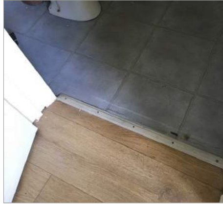
Photo - 42 Damage to cloakroom floor
